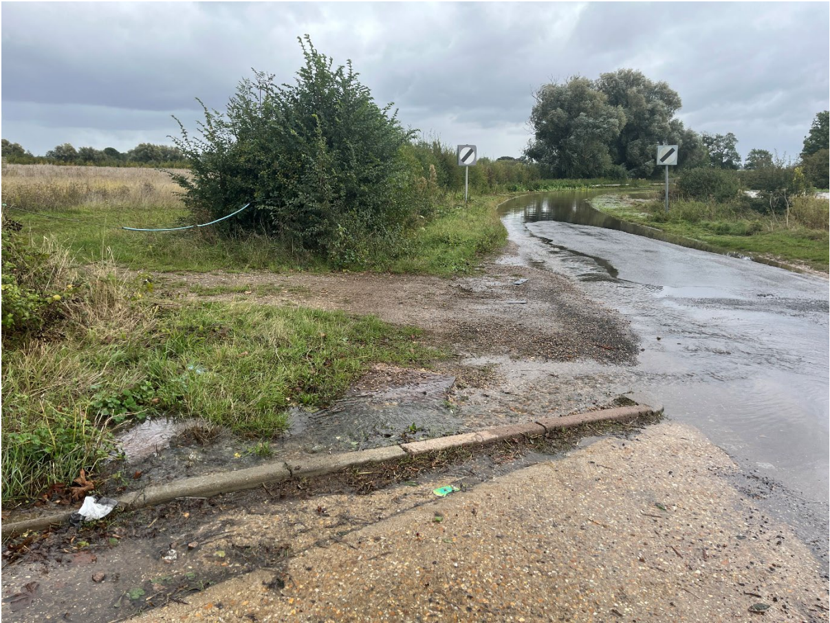
Taken on 27 th September 2024 of the flooded Great Staughton road by the small sewage works in Pertenhall.
